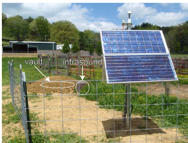
Figure 1-3. Photo of station TA.W52A (Murphy, NC), with solar panel assembly in front of an infrasound sensor cage and buried seismometer vault.
