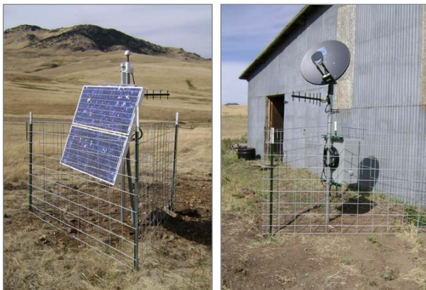
Figure 2-10. TA.D16A, a site with AC VSAT and radio relay to the station.
