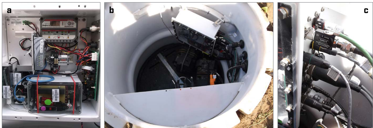
Figure 2-7. (a) Vault interface enclosure unit with lid removed and (b) as installed within vault (TA.L62A), with (c) close-up on the connectors (TA.D60A).
