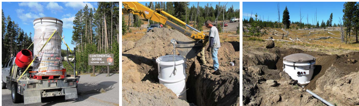
Figure 2-4. Construction of TA.H17A, Yellowstone National Park. The site used the second generation vault.
