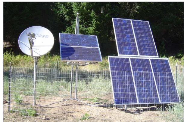
Figure 2-11. TA.N02C, a site with DC (Solar) VSAT
