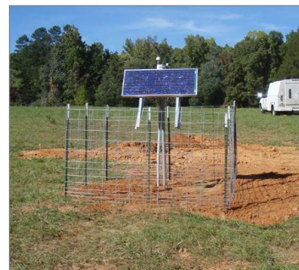
Figure 2-9. TA.KMSC, a site with good skyview and cellular telemetry only requires a single panel.
