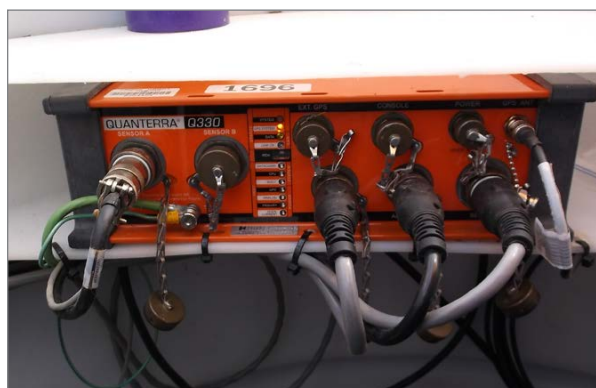
Figure 2-27. Typical Q330 installation, TA.D56A.
